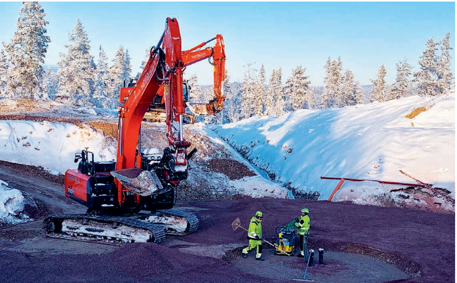
Work on a wind turbine foundation at the Åndberg wind farm (286 MW) Photo: OX2
