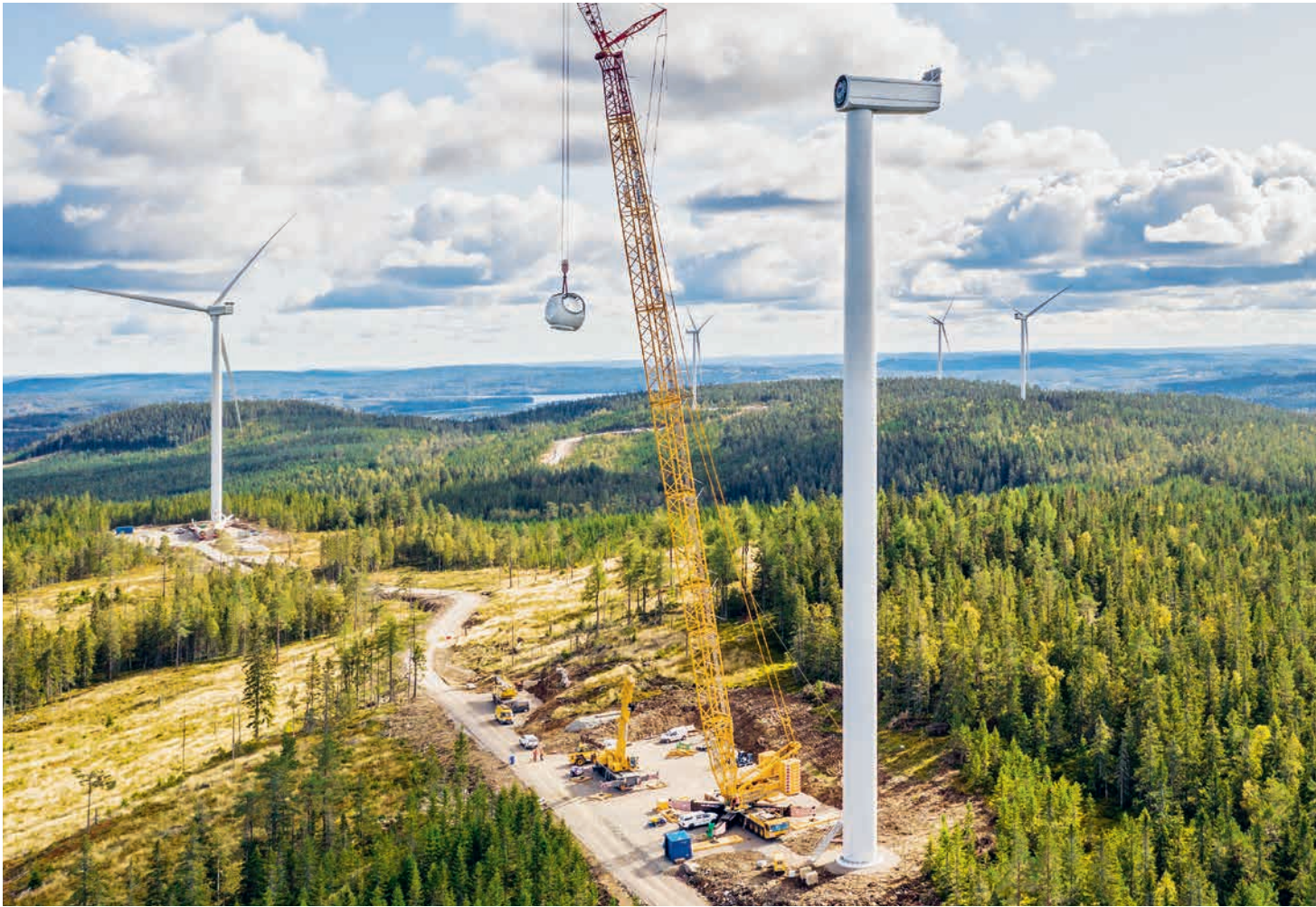
Construction of the Orrberget wind farm (33 MW) in Sweden. Photo: Joachim Lagercrantz
