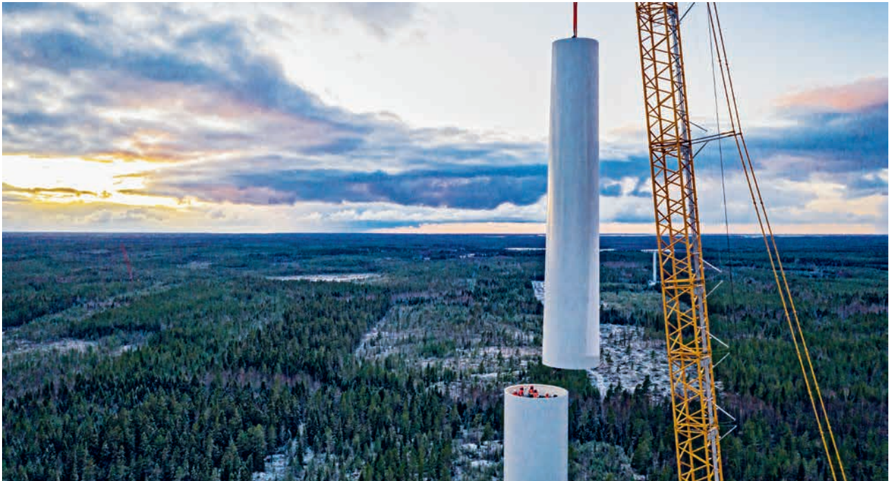
Construction of the Långmossa wind farm in Finland. This wind farm is part of the "Castles" project (107.4 MW). Photo: Joachim Lagercrantz
