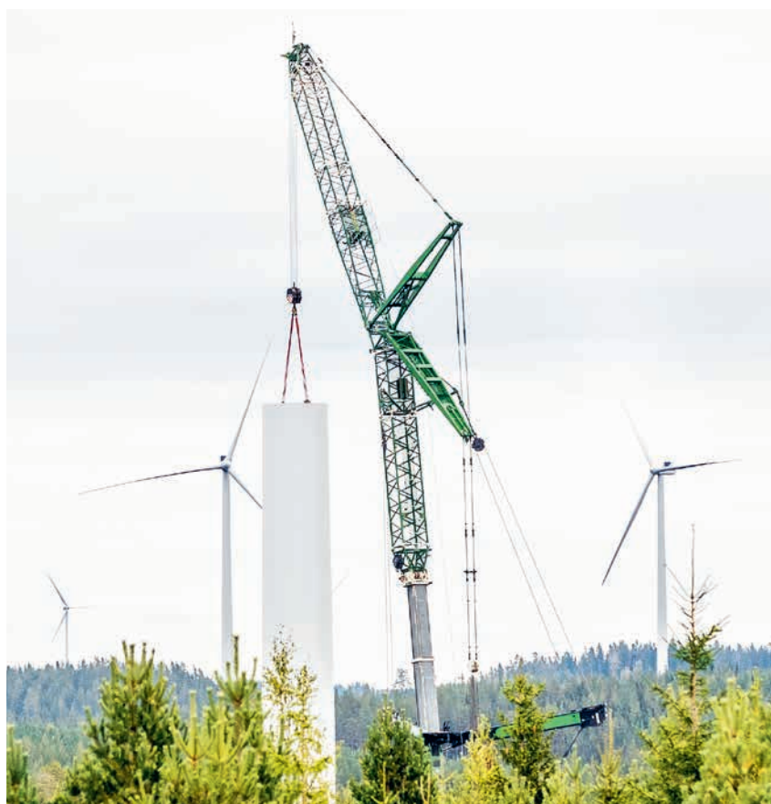
Construction of the Åmot-Lingbo and Tönsen wind farms (366 MW) in Sweden. Photo: Joachim Lagercrantz
